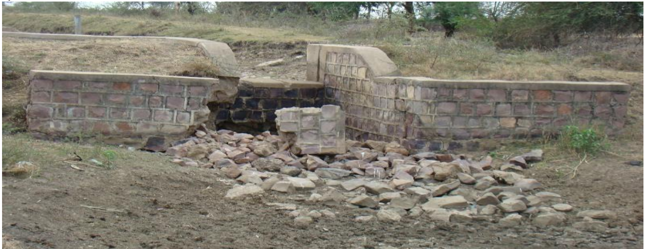
Photo 1 State of a Fall in the distributory at Tawa
